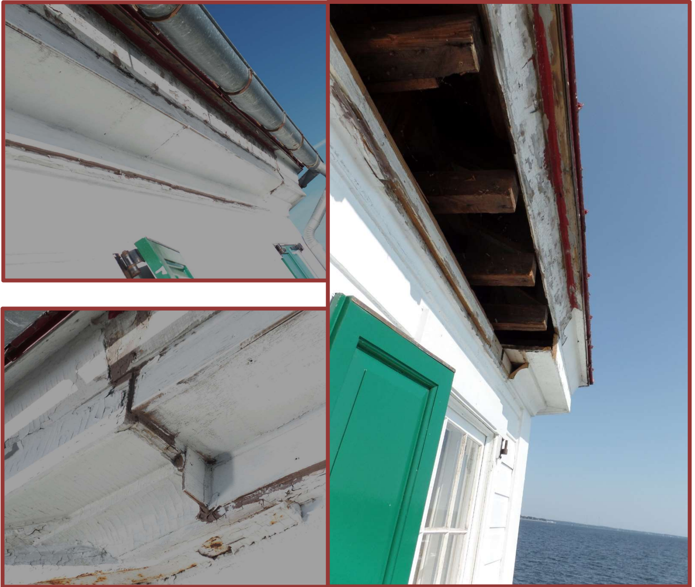
Soffit with water damage and missing cove molding
